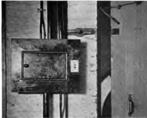
Fig. 3. Emergency Light for Stairway. (Eastman Kodak Company.)
